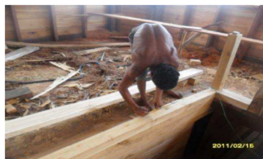
Figure 2 Process to make exterior
